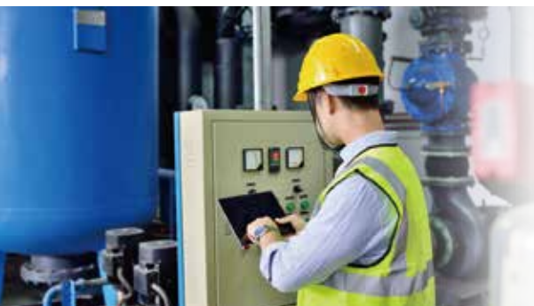
Control panels at industrial plants
